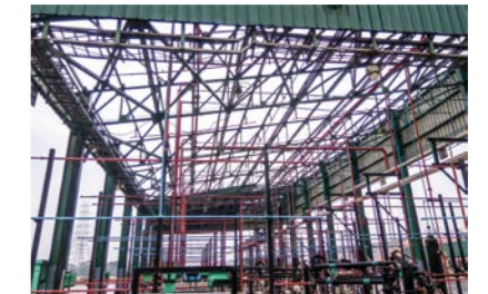
GONE WITH THE WIND The roof of the filling plant was no match for the cyclone
