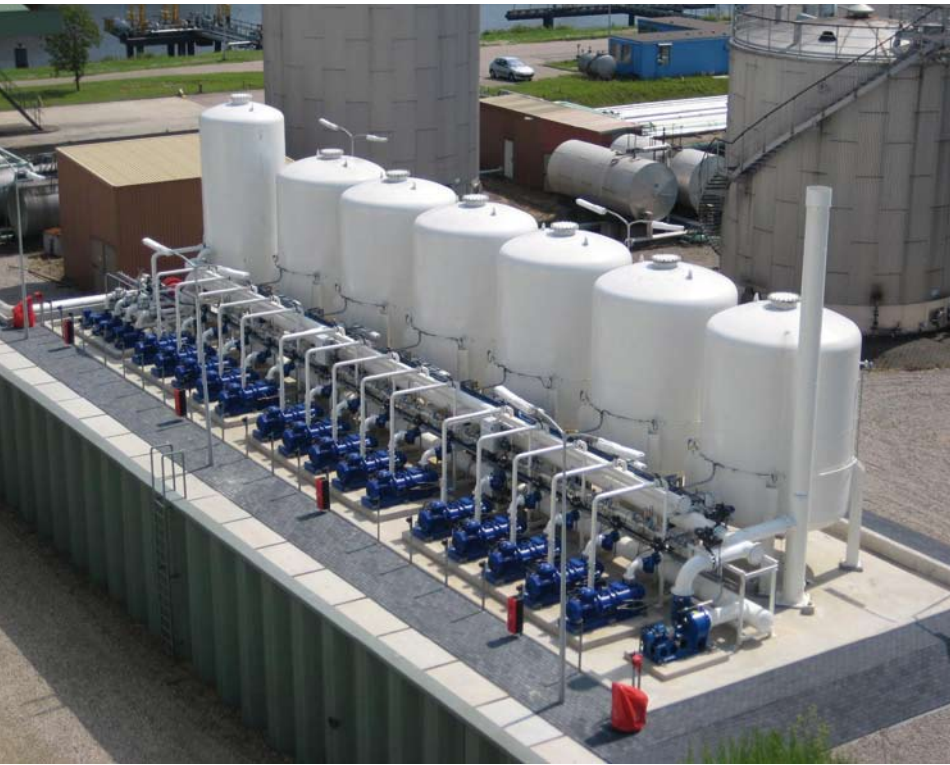
PARAGON The ultra-modern technology used by the new vapor recovery unit (VRU) at the Oiltanking terminal in Amsterdam.
