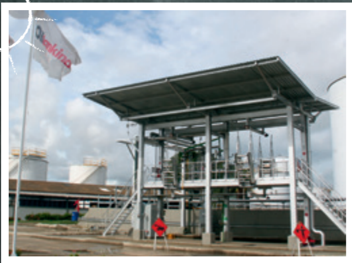
Solar Energy System Cartagena, Colombia
