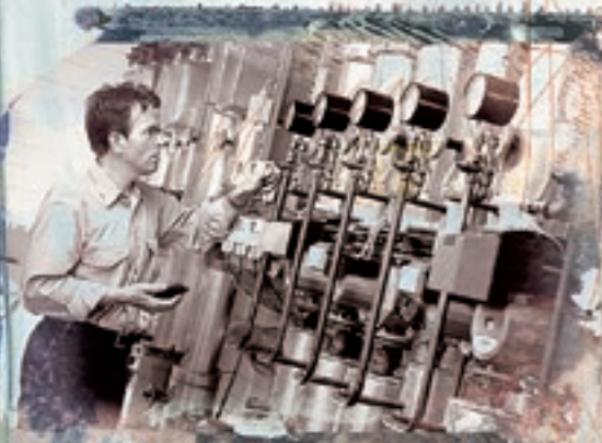
Noon, Proenergy, Bochum, Germany. An engineer inspects the heating systems by checking the eBox.
